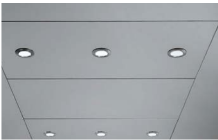
Ceiling lighting - standard LED round spot downlights
